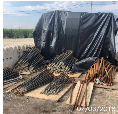
2.3.3 Metals and other materials isolated from the ground, to prevent soil contamination.
