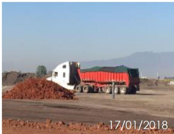
2.1.2.5. All trucks loaded with materials arrive at the project with protective tarpaulins.
