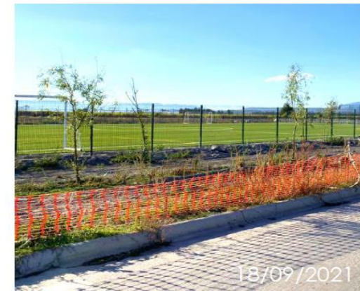
2.1.2.7. The construction team kept the future garden areas clean, avoiding pollution from garbage, debris, construction activities and machinery use.
